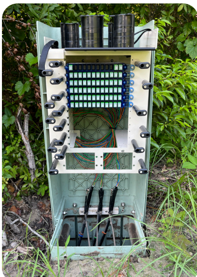
The PON bulkhead is in the FiberFirst Pedestal.
